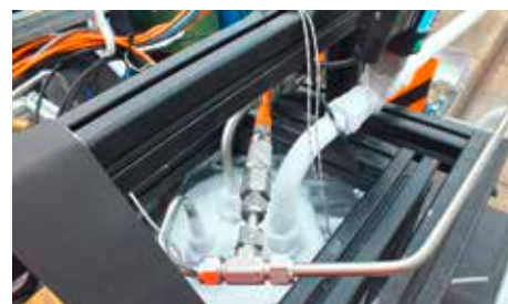
Ice on the main line to the machine.
