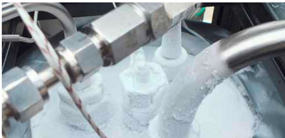
Significant amounts of frost showing on the top of the liquid oxygen tank. These are the conditions the O-ring has to cope with.
